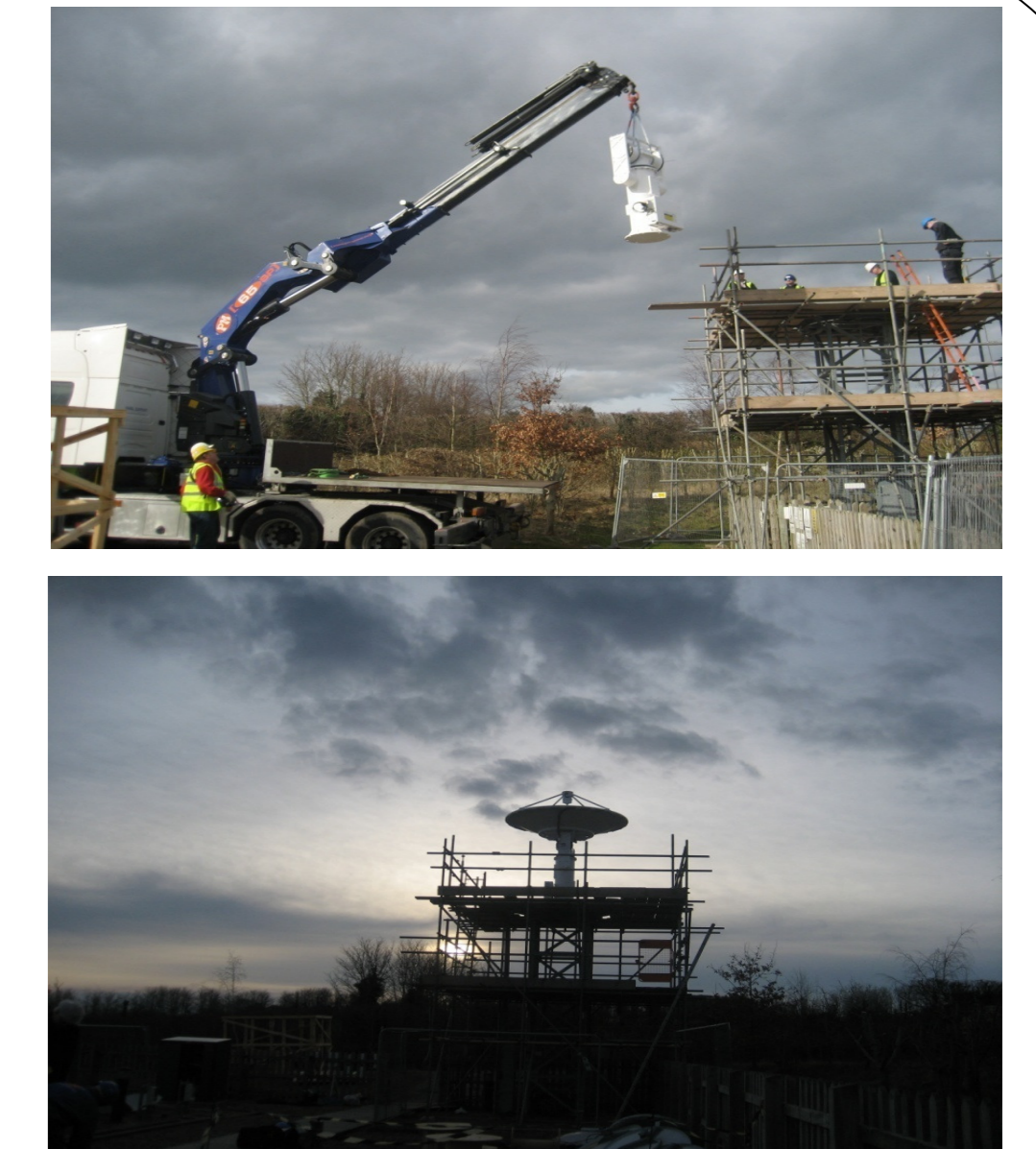
Figure 2. Upgrade of the Met Office direct broadcast reception facilities at Exeter HQ. Our two polar orbiting satellite tracking antennae were upgraded to enable X-band reception specifically for the reception of Suomi NPP data.
